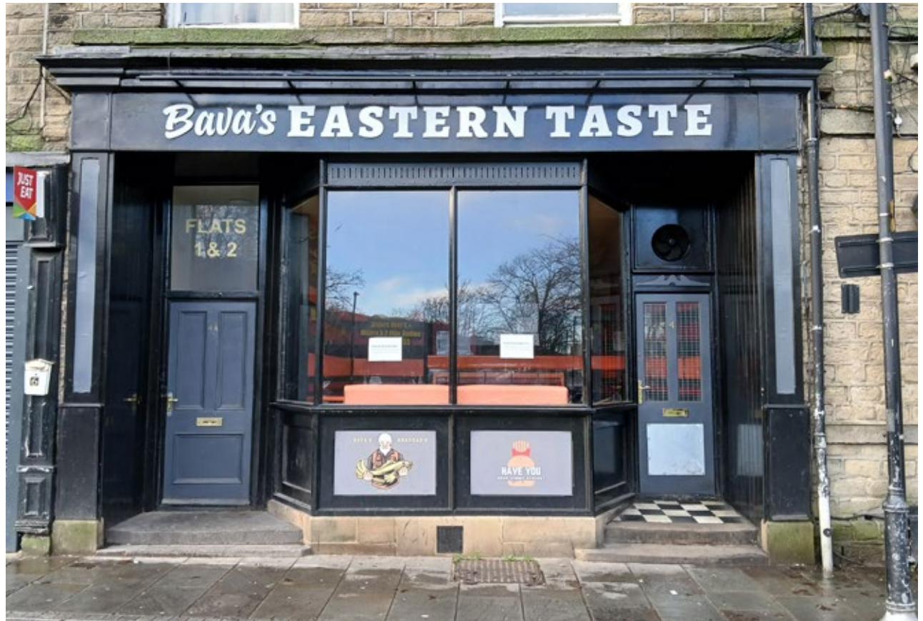
Discretely incorporated ventilation above the shop windows on Church Street, Keighley
