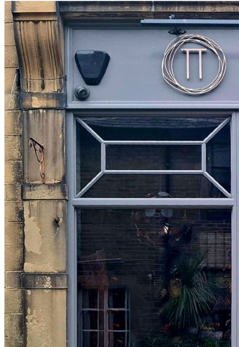
Well-positioned and colour coordinated alarm boxes and CCTV cameras ( Haworth )
