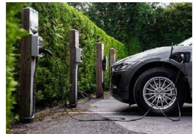
Figure 25: Public electric vehicles charging points
