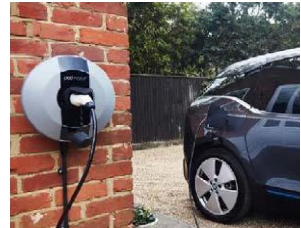
Figure 56: A public electric vehicle charging point in Tickhill, South Yorkshire.
