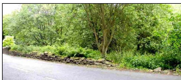
Collapsed dry stone wall, Denholme Road.
