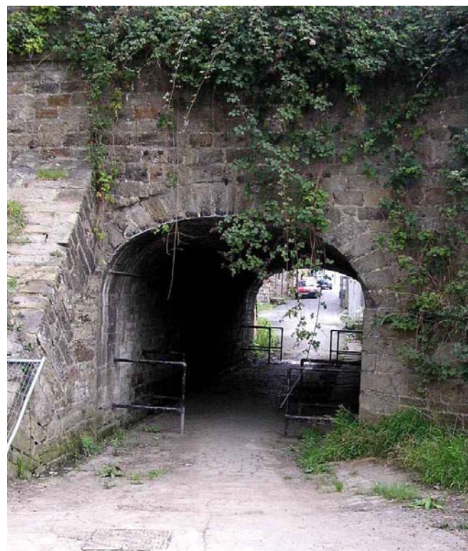
The canal is carried over Hainsworth Road by Silsden aqueduct (Grade 1 Listed). Expensive pieces of engineering such as this are typical 'Brindley features' of canals where John Brindley was employed as engineer. The aqueduct is in need of better maintenance.
