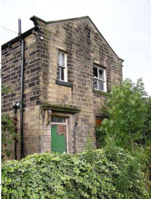
2. High Bank House currently stands empty and in a deteriorating condition.
