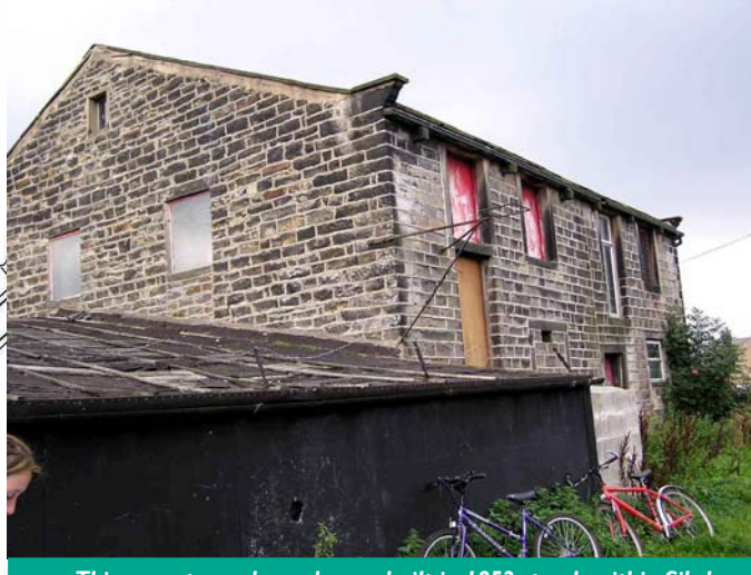
This vacant canal warehouse, built in 1852 stands within Silsden conservation area and is in need of a sustainable new use.
