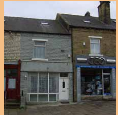
Vacant building, painted elevation and modernised shopfront all inappropriate features.
