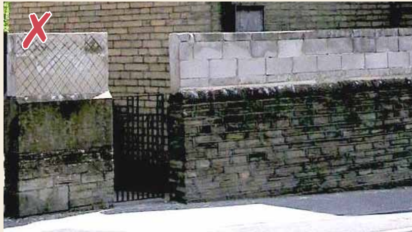
Figure 51: Poor quality and unacceptable addition to stone wall
