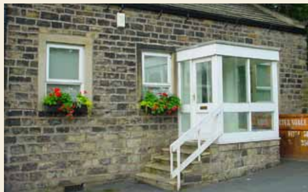
Figure 24: Large and poor quality porch not acceptable
