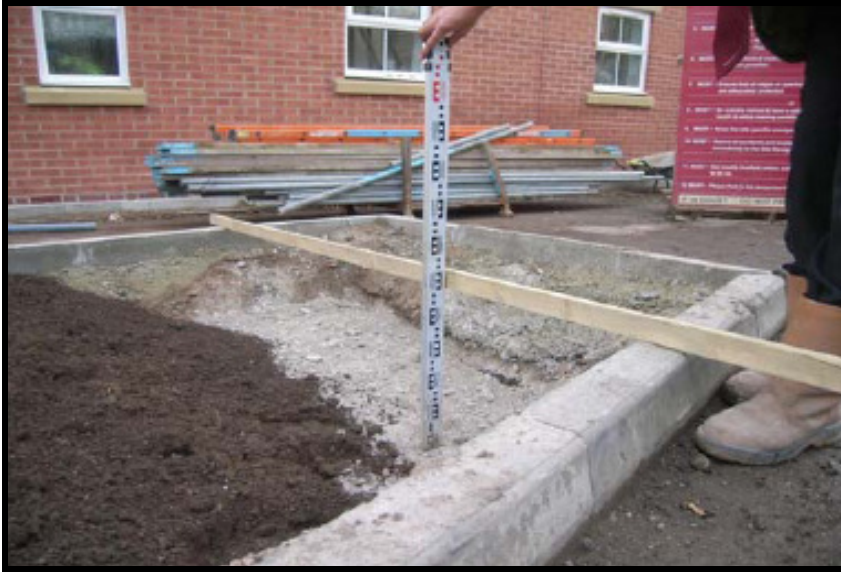
Photograph 1 : Depth check of inert cover within area of public open space. Physical break layer and topsoil visible.
