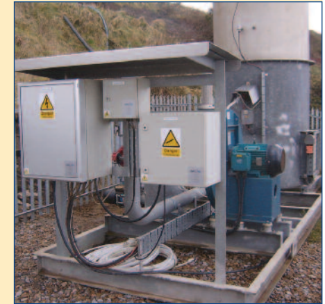
temporary gas flare equipment
