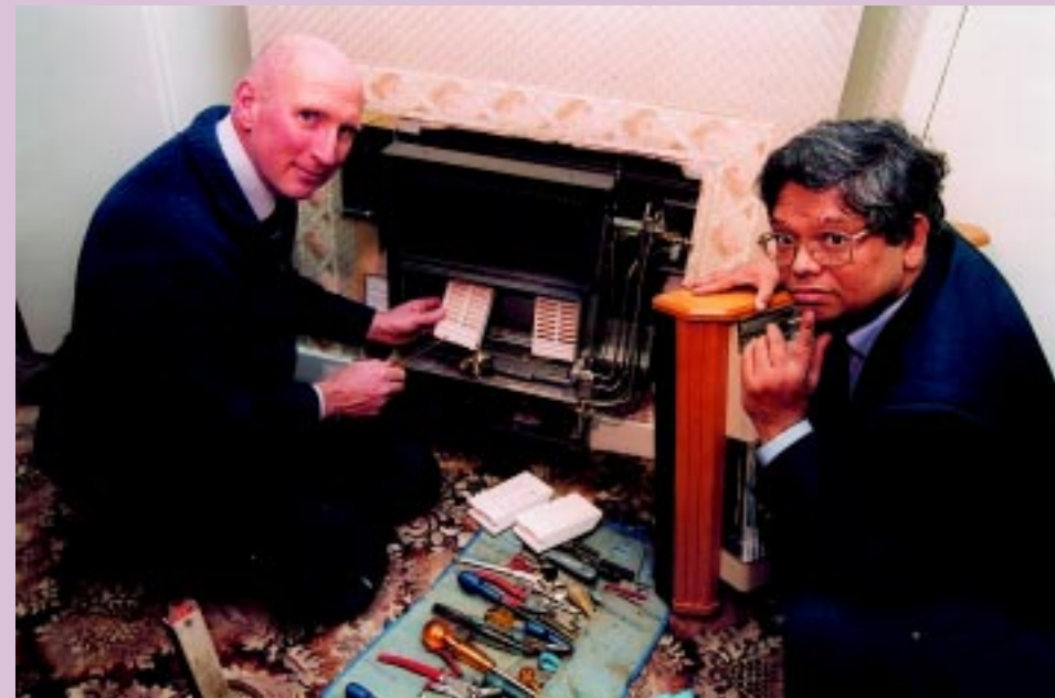
Left, a landlord gets gas appliances checked in his property in time for a new tenant
