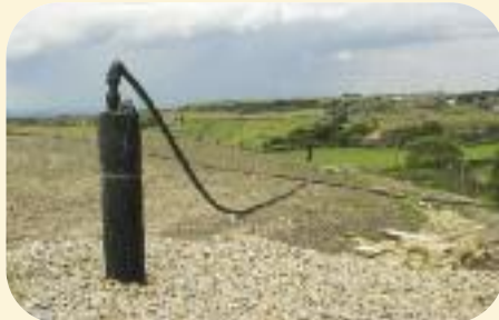
Top of new borehole with gas extraction pipe, surface water drainage gully and view East.
