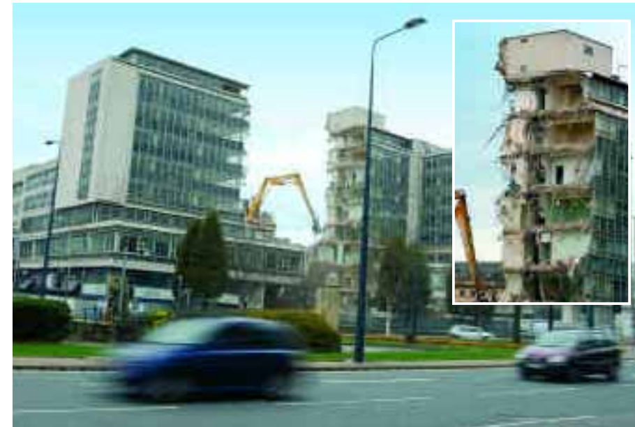
Nibble by nibble the jaws of a 100-foot crane have eaten into Forster House as demolition makes way for the Broadway development in the city centre.
