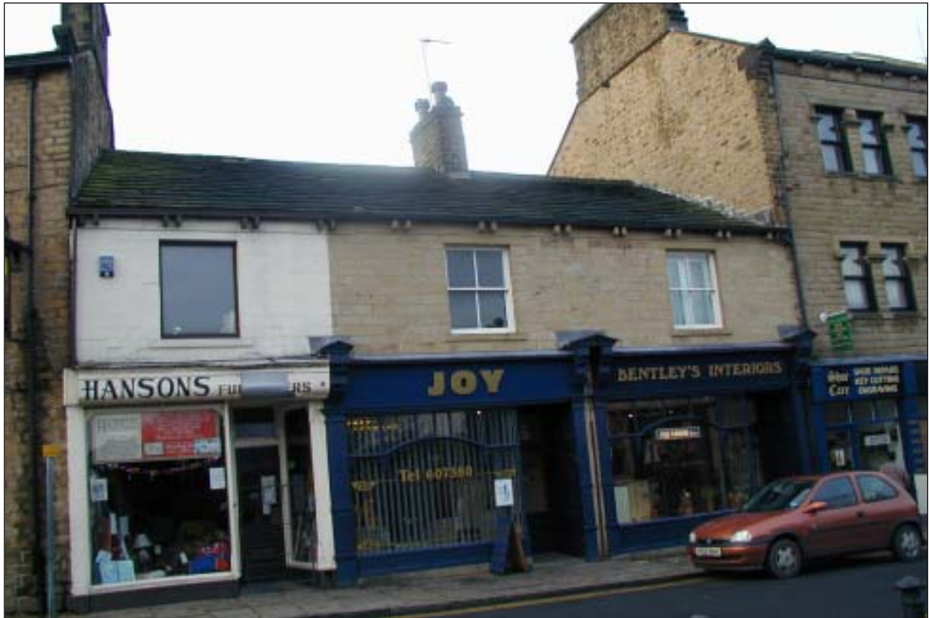
10, 12 and 14 Church Street – with their traditional shop fronts and 4-paned sash windows. Changes such as painting or inappropriate replacement windows can destroy the unity of a group of buildings such as this terrace.
