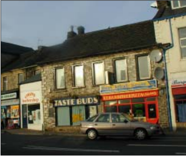
40 –42 High Street (Grade II) – considered to be the oldest building in the conservation area, but sadly disfigured by the insertion of unsympathetic shopfronts and out of scale signage. The first floor windows lack traditional features.
