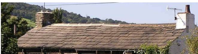
Top: These well maintained chimneys enhance the appearance of this house. Above: The removal of posts and cornice detail and the shortening of the stacks has drastically altered this roofscape.
