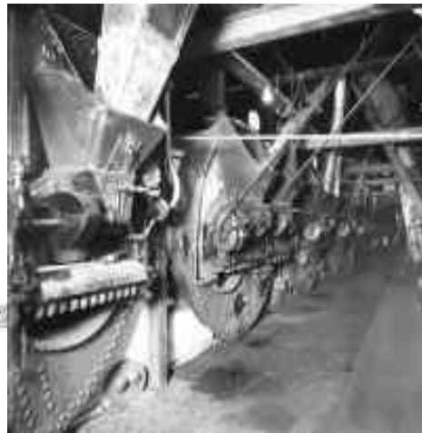
Underground installation of boilers, shafting and belting was designed for Salts Mill with the aims of providing a safer working environment and an integrated approach to the production of textiles. Source : RCHME
