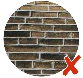
This smooth cement rich mortar contrasts with the stone of the wall. This is compounded by its application as strap pointing which stands proud of the stone.
