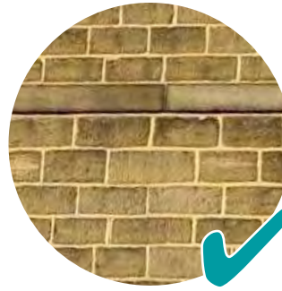
The mortar is of a sandy colour and texture and has been applied within the joints only to give a traditional look to the wall.
