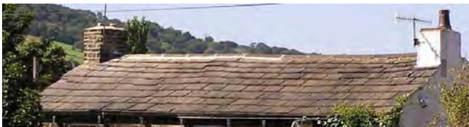
Top: These well maintained chimneys enhance the appearance of this house. Above: The removal of posts and cornice detail and the shortening of the stacks has drastically altered this roofscape.
