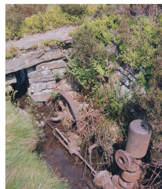
Water pump at marker 10
